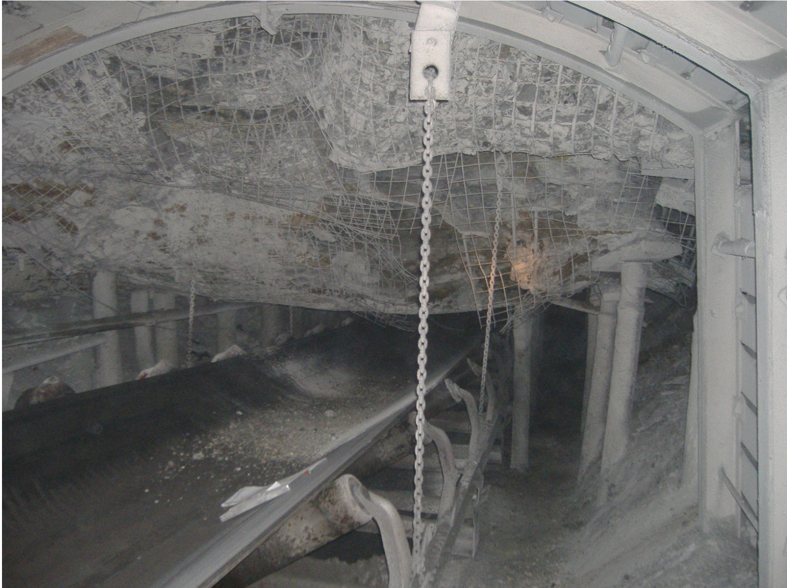
Bailey Mine main line haulage roof and rib deterioration over 20 years.
