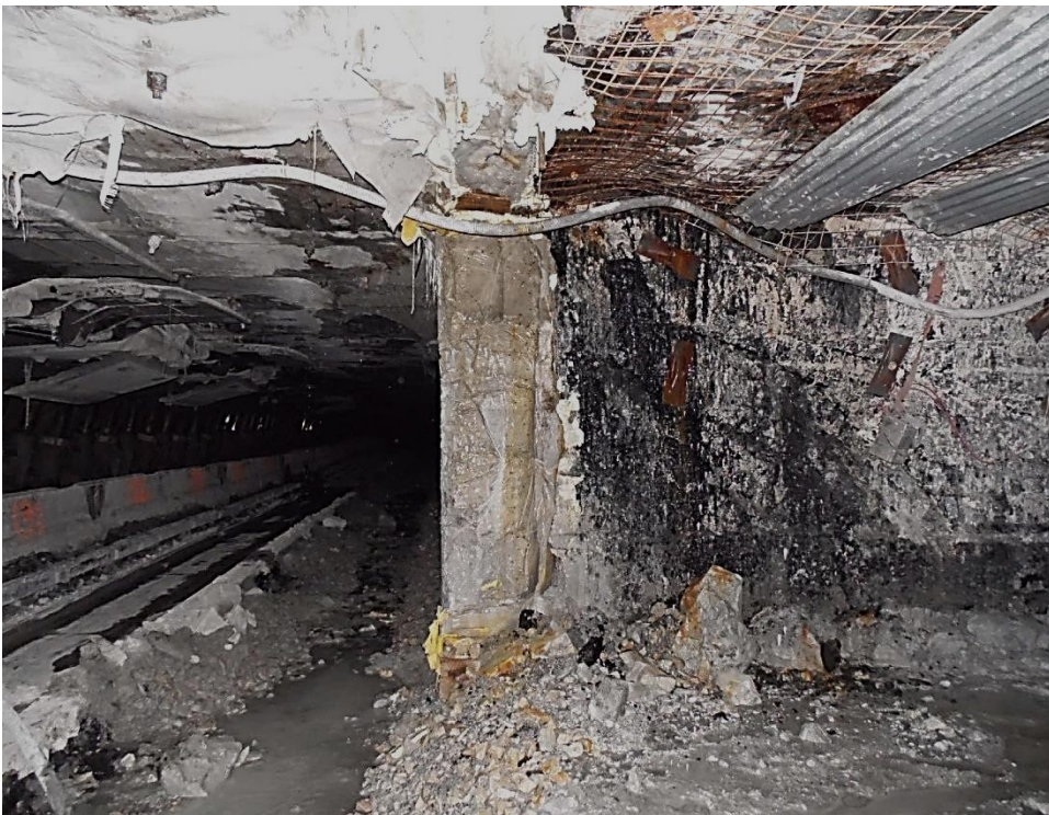
Breakthrough to chute 4, some spalling. The face is standing straight.
