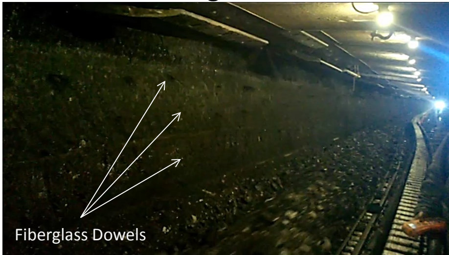
Mining the coal fender approx. 5 feet of backfill. The fender is standing straight.
