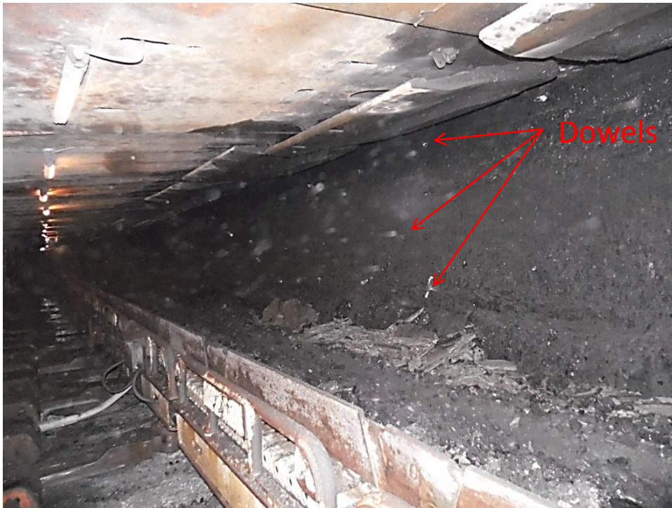
Mining the coal fender, no roof spalling. The face is standing straight. Mining within 13 feet of the backfill.
