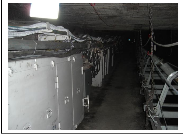
Figure 11. Monorail-Mounted Emulsion Pump
