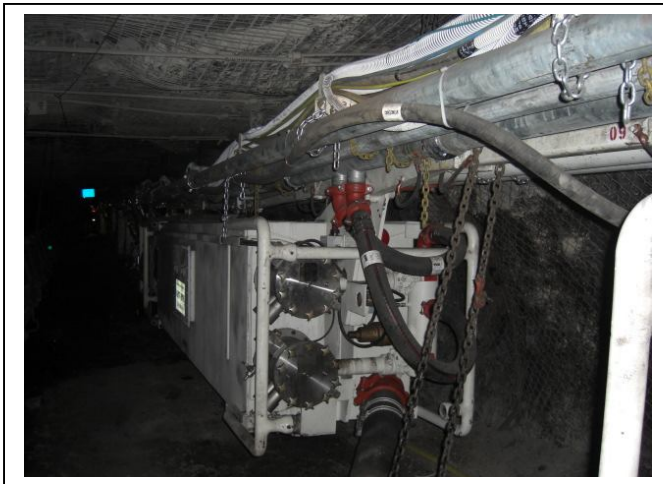
Figure 12. Monorail-Mounted Emulsion Tank
